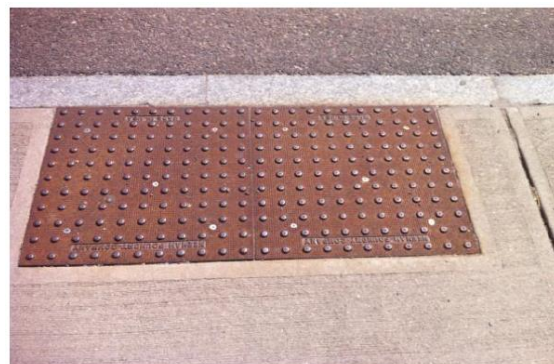
Figure 2. VTrans Cast Iron DWP (Installed 2005, Photo 2013)
