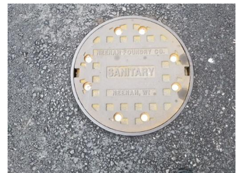
Installed 1772 manhole cover with new venting (courtesy, City of Fort Wayne, IN)
